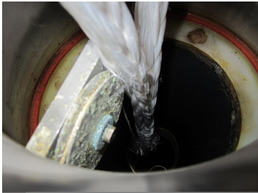
Figure 4.2: Photograph showing corrosion to one of the pulleys of the equator-monitoring system.
