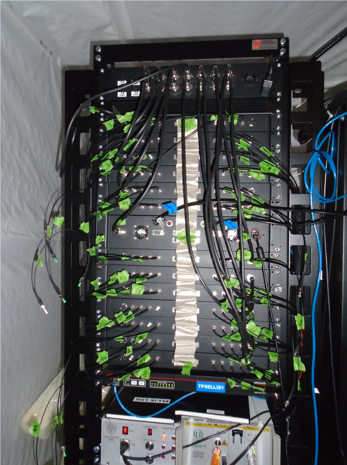
Figure 3.24: A photo of the TELLIE rack. The control box is in the middle. Two ribbon cables are connected to the control box, one connects to 7 TELLIE driver boxes below it, other one connects to 5 TELLIE boxes and 1 AMELLIE box above it. A power box is at the very top, distributing power to all other boxes. Green tags are marking the optical fibres, with their corresponding ID number. The numbering ensures that the fibres are re-plugged to the correct channel output, if they need to be unplugged. Blue tags mark trigger-in and trigger-out cables. The USB interface cable is also visible connecting to the control box.
