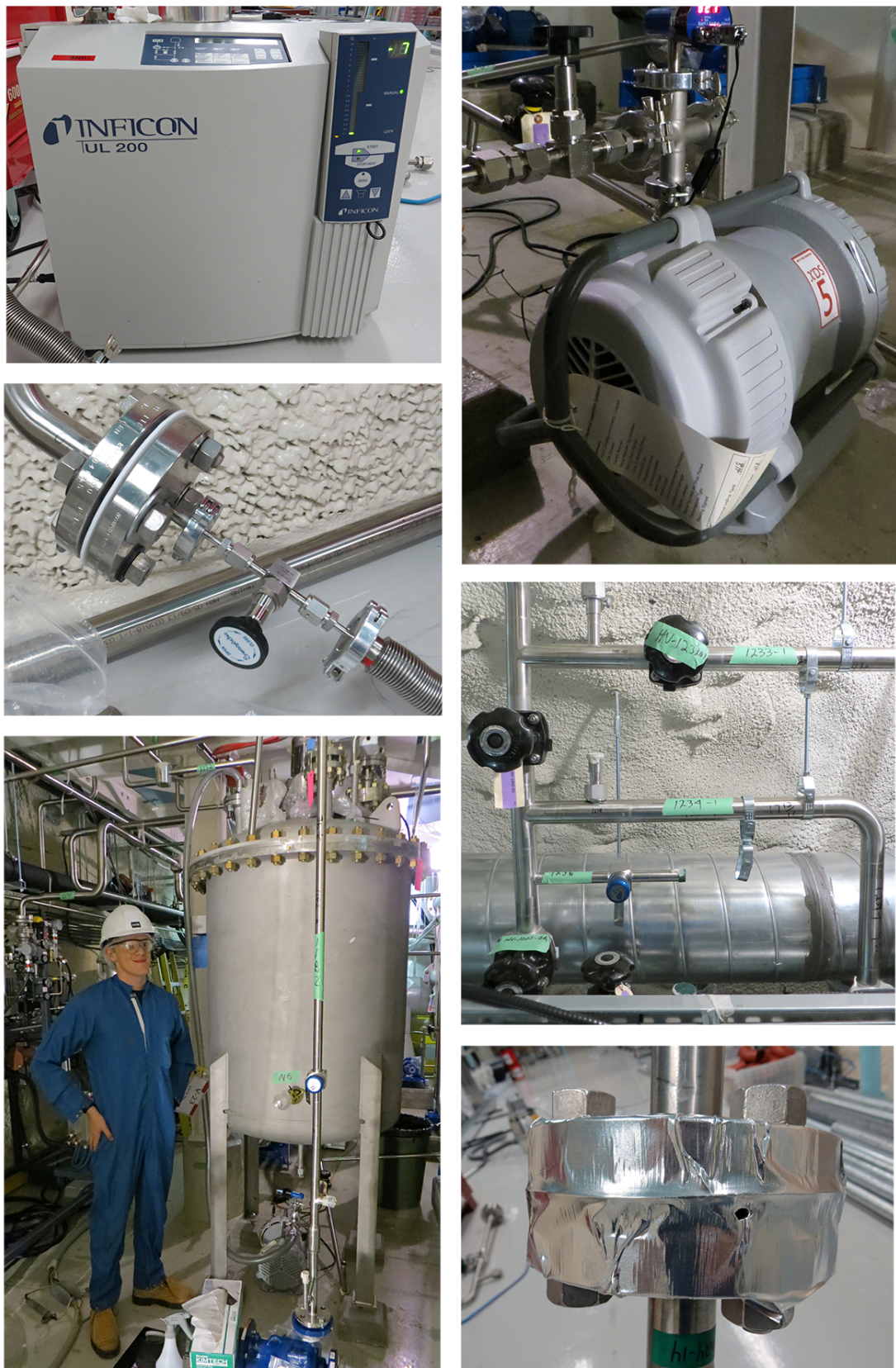
FIGURE 3.21: Top-left: helium leak detector and vacuum pump. Top-right: scroll vacuum pump. Middle-left: needle valve. Middle-right: pipelines and hand-valves. Bottom-left: author beside vessel. Bottom-right: joint sealed with aluminium tape, a hole is pierced in order to inject helium.
